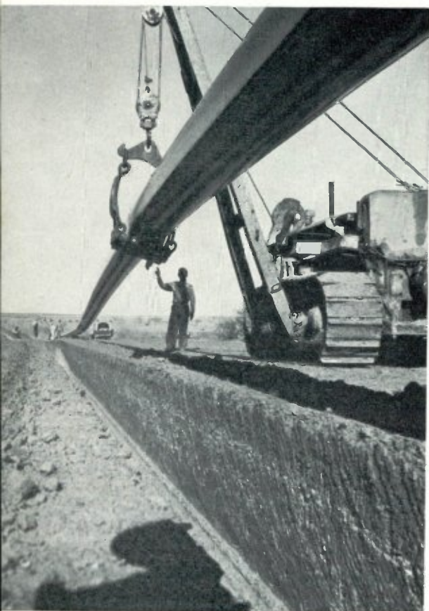
A new pipe is lowered into its trench. It will carry crude oil from Jal, N. M., to Wood River, Ill.
