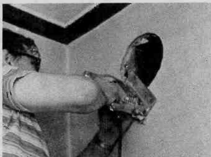
Fig. 4. If you have made a measuring error and find a stud running past the hole, don't panic. The wall will stand even if you cut through one stud. Use a saber saw to trim the stud so the cuts correspond to the circular duct pattern.
