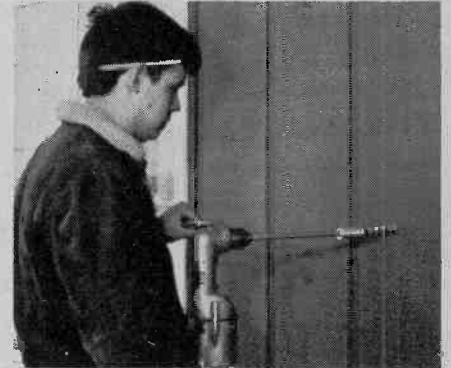
Fig. 23. A hole is drilled immediately below the patio speaker at the site of the remote control unit.
