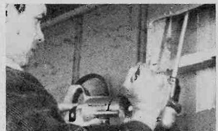
Fig. 21. An extension drill is used to drill a hole into the attic. This drilling procedure was necessary because it was difficult to drill a hole down from the attic. Once hole is made, pull down cable from attic.
