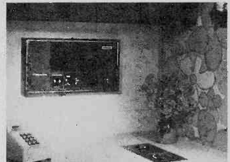
Fig. 19. The master control station is flush-mounted on its rough-in frame and secured in place. What was once a hole in the wall is now the mark of a professional-like installation you can do.
