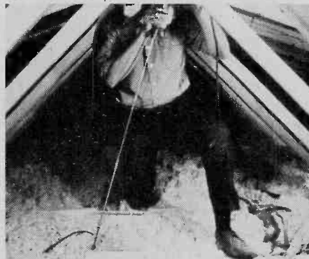
Fig. 3. Once in a while you'll run into a tough one. A fire stop in an unusual location may require a shifting of location of a remote station, or the renting of special tools to do the job. This homeowner rented an extension drill to go through a fire stop in the wall below that was troublesome.
