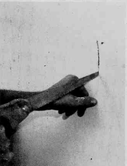
Fig. 10. Use a key saw through wall board, dry wall (sheet rock), and the like. Pilot holes drilled in the corners give the key saw a starting point. Saber or jig-saws may be used. Plaster walls require special treatment as described in text.
