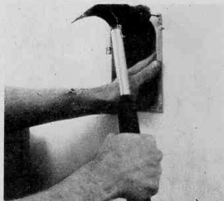
Fig. 11. If you did a good job cutting out the hole, the rough-in frame should fit snugly. Tap the frame in place, then nail one edge to the wall stud.
