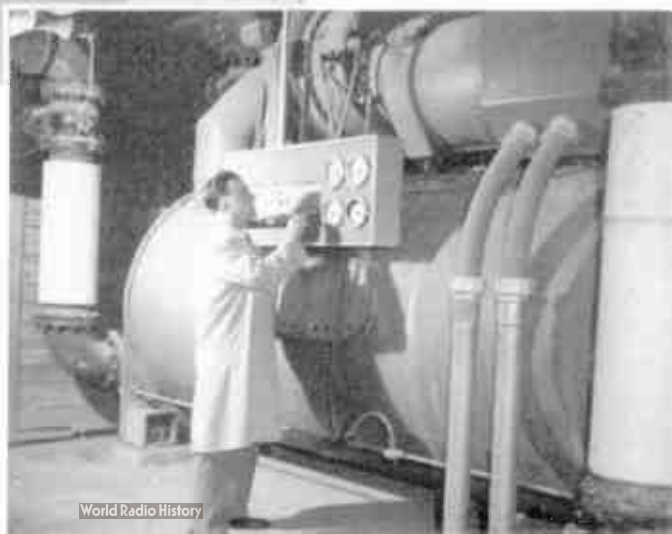
Building Superintendent Chris Fitzgerald checks electronic control panel on one of three 500-ton York Turbopak refrigeration compressors in basement.
