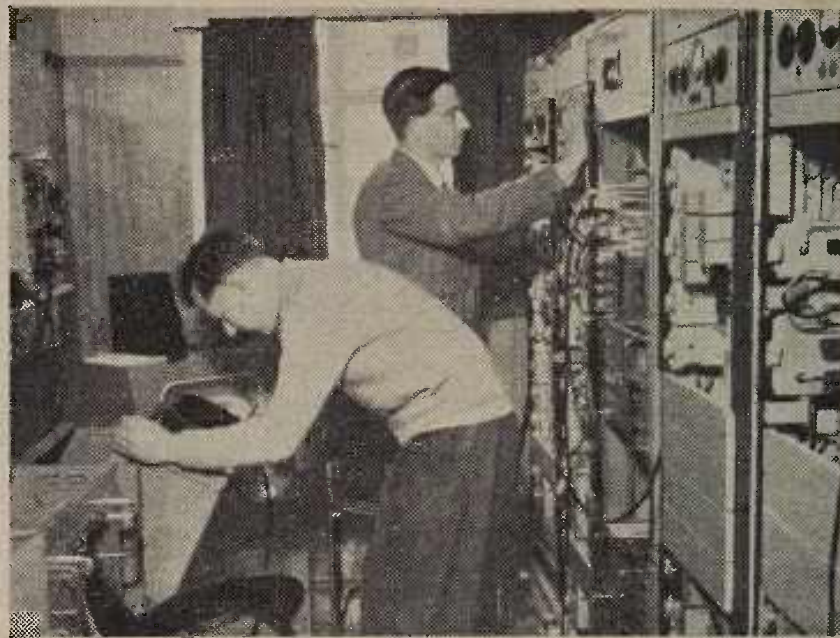
Some of the equipment at one of the repeater station.
