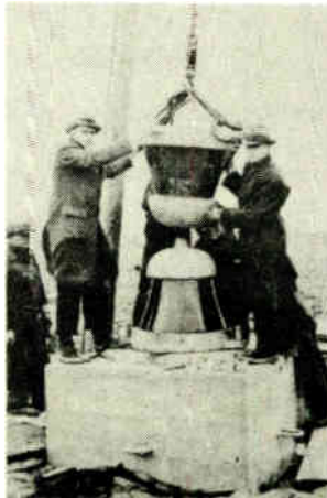
Placing Base Insulator which would eventually, and to this day, support 110 tons of steel and 340 tons of guy pressure.
