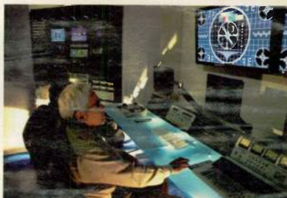
Fully Functional Master Control Room- LA Showroom
