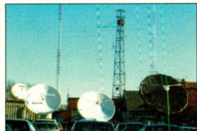
WCVB-TV's MRC omnidirectional receive system is installed on a 100-foot tower at its studio location.
