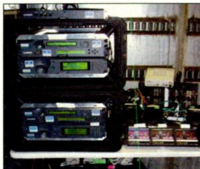
One of the Tandberg Television encoder packages used by RTM Remote Transmission Management
