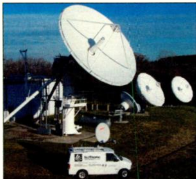
The Patriot Antenna Systems installed at the IsoTropic teleport in Geneva, Wis.
