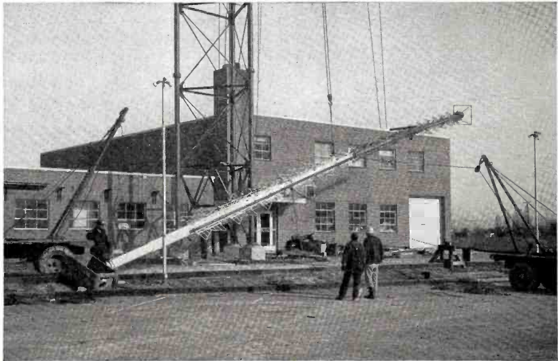
A TALLER TOWER...AND MORE POWER...FOR WXEL, CLEVELAND
