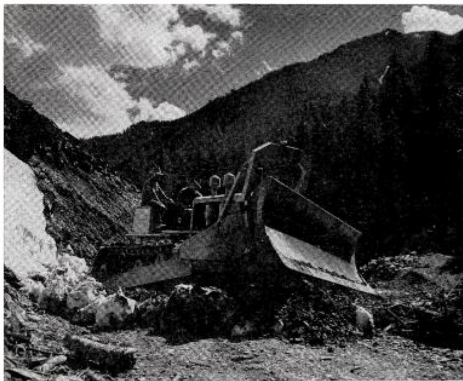
MOUNTAINOUS obstacles crumble before the might of a Caterpillar tractor as a new road is cut through some of the nation's roughest terrain. New and better roads plus deeper river channels and expanding air transport, are joining railroads in the effort to remove the Northwest's semi-isolation from the rest of the U. S.
