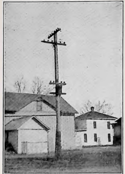
Fig. 6. Pole and Transformer in Pole-Line Distribution System
