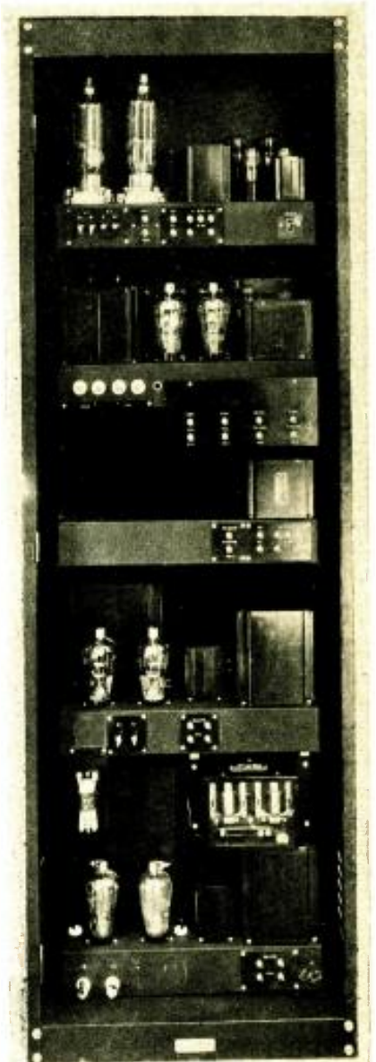
Rear view of the rack containing the power supplies for the entire transmitter, as well as the modulator.
