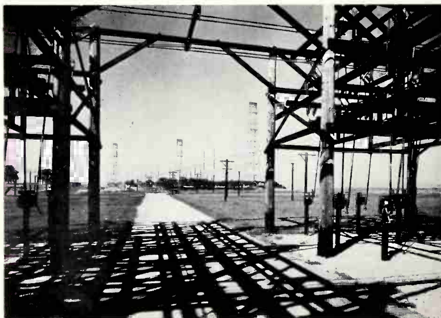
Shadows of some of the 20-foot poles in a forest of 232 switches which can be manually operated from the ground to connect any of the six transmitters with any of the 22 antennas of the VOA facilities at WLWO, are maintained and operated by Crosley Broadcasting Corporation as a relay base for broadcasts.
