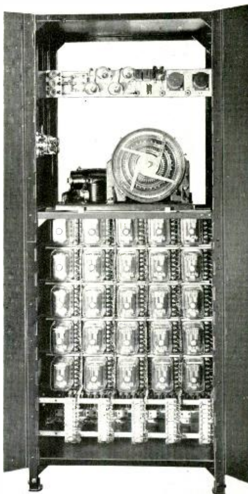
A typical distributor and relay assembly for either end of the system
