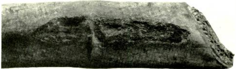
Fig. 2—Chemical attack due to alkali formed by stray current entering sheath
