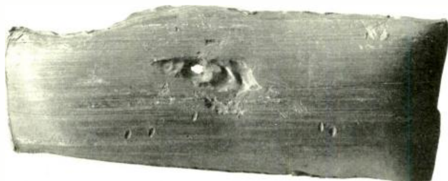
Fig. 1—Electrolytic corrosion due to current leaving sheath
