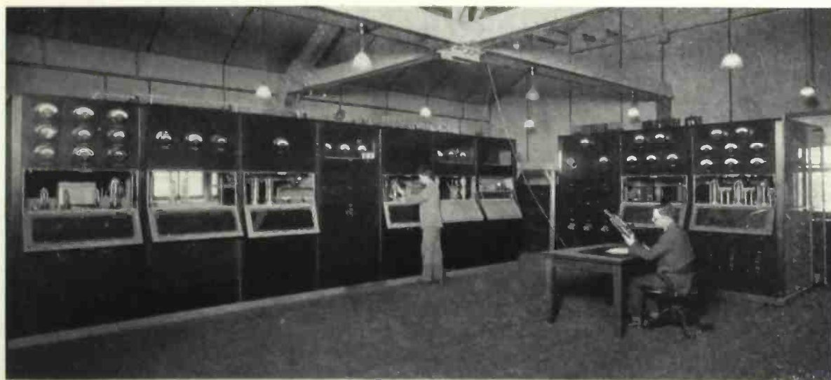
A general view of the transmitter room at Whippany
