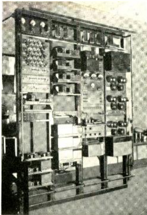
Fig. 6—Carrier panels in typical repeater station
