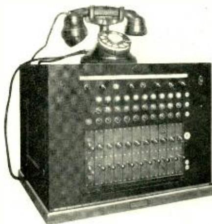
Attendant's cabinet, located in a butler's pantry. The pictures were taken at the first installation, on a large country estate
