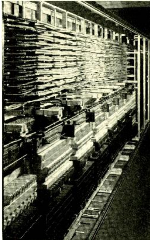
Fig. 2—A rear view of the new board shows the compact grouping of the relays on their steel supporting structure and the accessibility of the multiple
