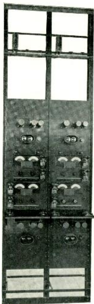
Fig. 2—Two bays of panel-mounted terminal equipment, equivalent to a single bay new equipment
