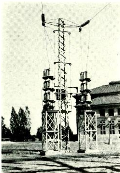
Fig. 3—Coupling condensers for 110,000 volt lines
