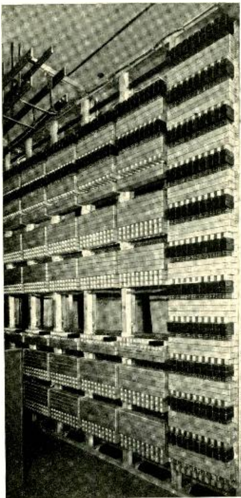
Fig. 4—Incoming trunk, overflow, and idle-line indicating equipment in shop wired units is mounted on relay racks
