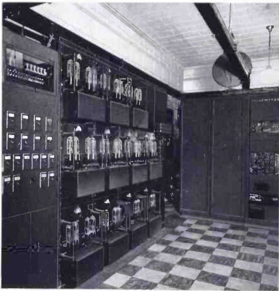
In the control room are also the power amplifiers and their control racks
