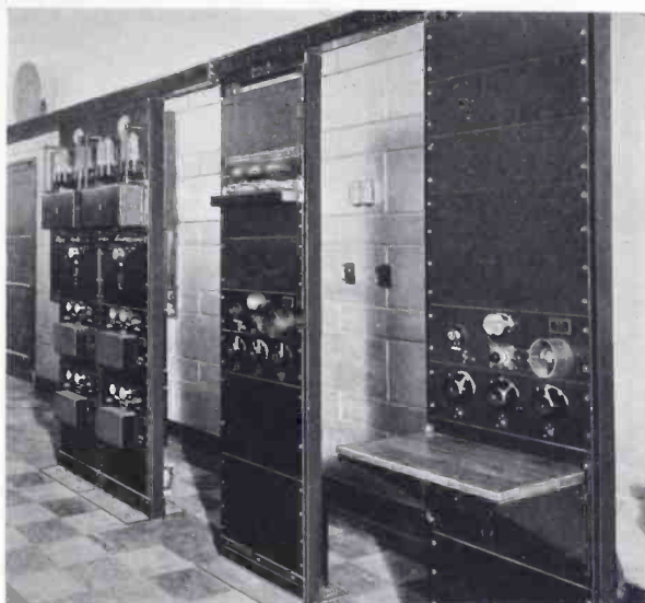
Programs transmitted to broadcasting stations are controlled from the two bays at the right. Adjacent to these bays are the two speech-input bays for the public address systems of auditorium and ballroom
