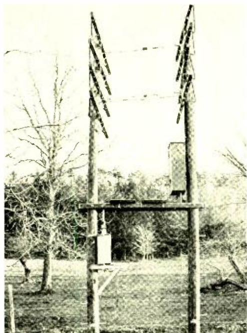
Fig. 2—An actual installation of a neutralizing transformer
