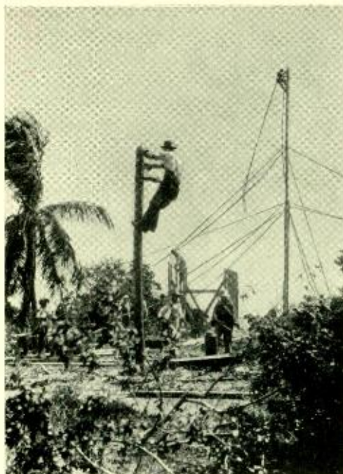
Space had to be cleared in the mangrove jungle before construction could start
