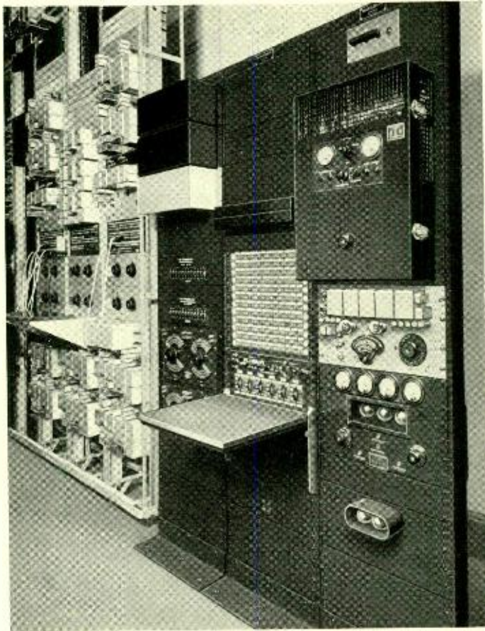
Fig. 2—Photograph of special equipment provided at San Francisco for overall tests
