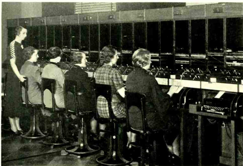
The No. 3A Switchboard which is now installed in about 30 centers, provides capacity for about 1400 subscriber lines and 240 inter-toll trunks
