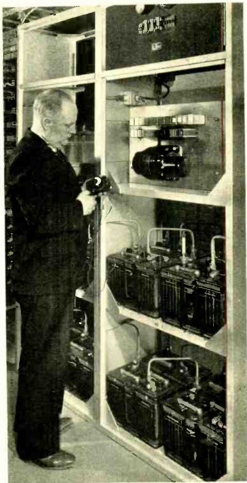
Fig. 2—The 105A power plant provides a compact unit for the smaller central offices and private branch exchanges
