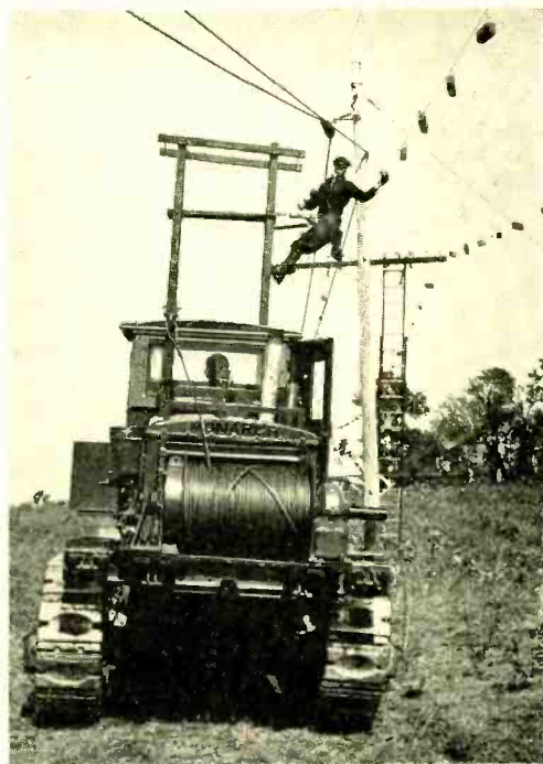
Fig. 3—Bricks hung on open wires to simulate ice load in line-wire tie tests
