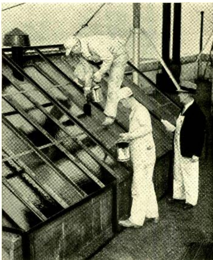
Blacking out a skylight on top of the West Street building. Left to right—Walter Gillis, Thomas Dorsey, and Thomas Solan, supervisor of the Plant Department's paint group
