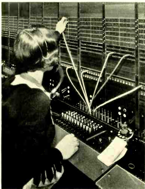
Fig. 1—A special-service position of the 13D board showing the additional space at the front of the key shelf, and the number-checking test strips in the upper part of the vertical sections
