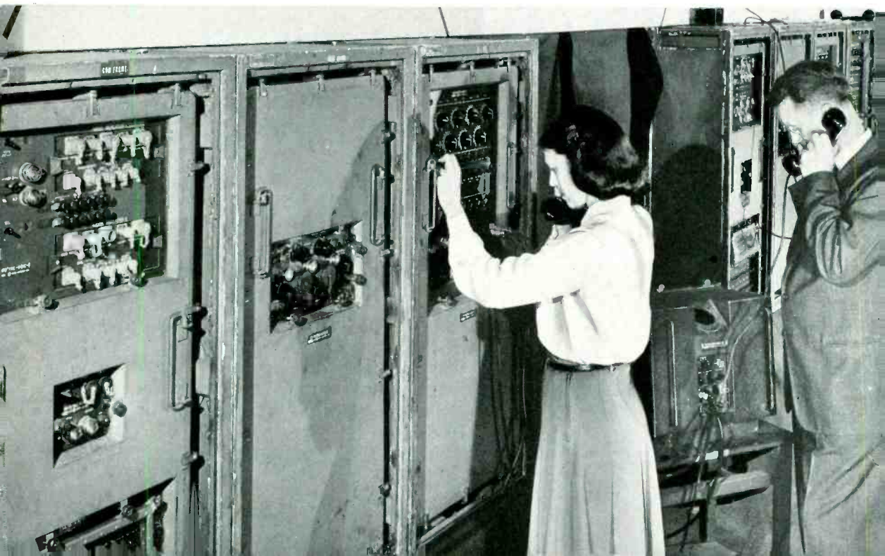
Three sets of AN/TRC-6 equipments in the "tank" room on the 32nd floor of the New York Telephone Building at 140 West Street
