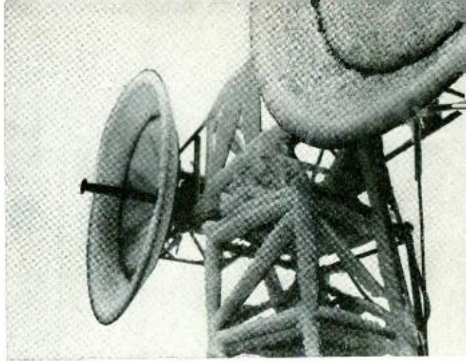
In the German mountains the antennas of the AN/TRC-6 system operated continuously with several inches of snow and ice on them
