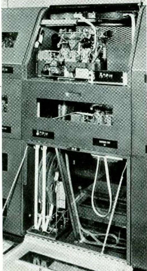
Fig. 3—Each cabinet houses two reperforator transmitters with tape storage space in the lower section
