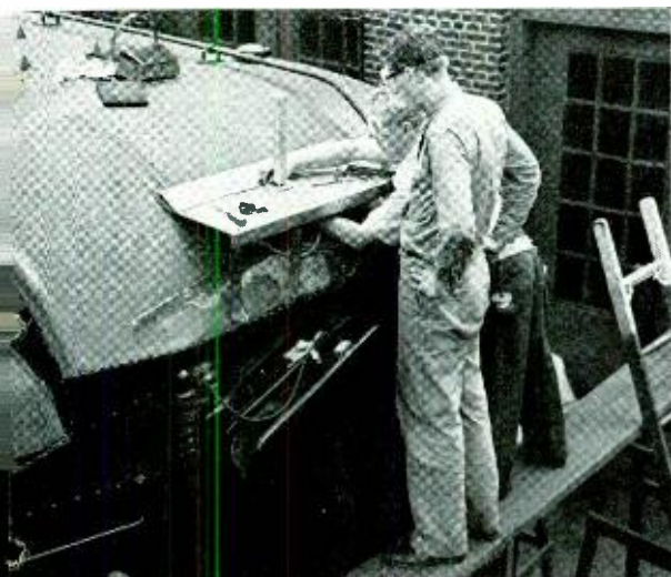
Fig. 5—Installing one of the antennas on the Pennsylvania Railroad lounge car "John Adams." J. L. Lindner, Bell Telephone Laboratories, at the left, and G. E. Goldner of The Diamond State Telephone Company
