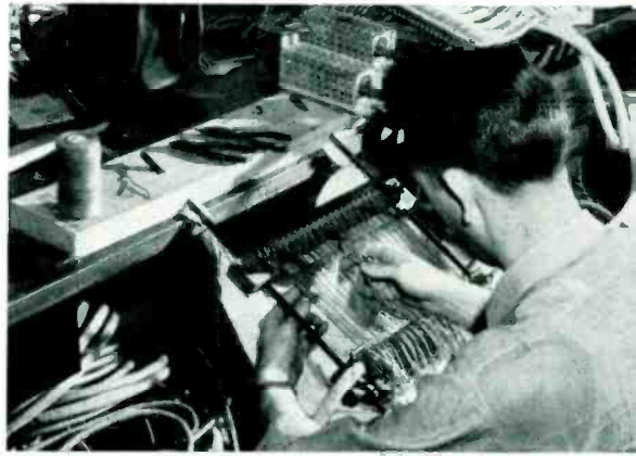
Western installer, J. F. Mulligan, solders new extension multiple jacks for a multiple run to be added to the Murray Hill 701A PBX
