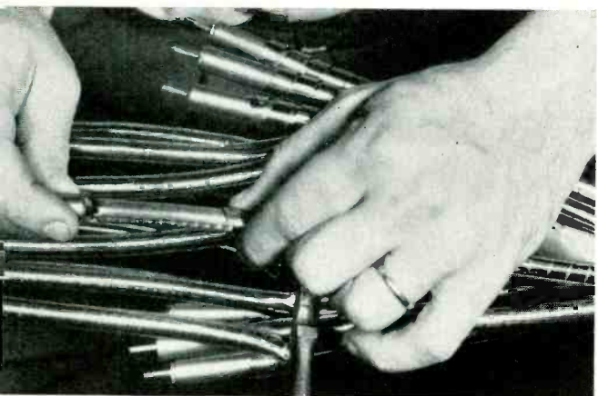
Fig. 3—A short copper sleeve is added to hold the steel tapes of the completed splice
