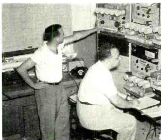
Test equipment in the AT & T repeater station at Madison. Left to right: L. A. Weber, and S. Korba.
