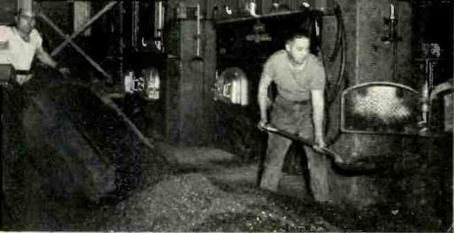
Cold weather means that more heat is required from the boilers. J. J. Moore fires boiler No. 8 while W. T. Quinn brings in coal.
