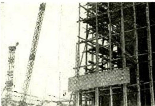
Contrasting construction methods in Berlin. On one side of the street, in the Eastern Sector, wooden poles are lashed together to form the scaffold. At the extreme left, in the Western Sector, a modern steel derrick and a concrete pouring tower can be seen.
