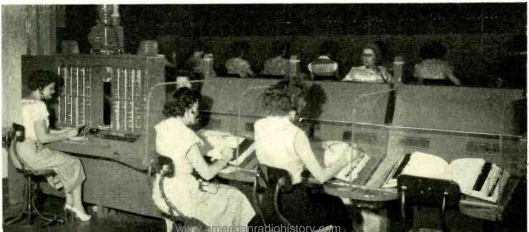
Fig. 6 – A 23D ticket filing and charge quoting section with pneumatic tube ticket distribution and three 23A sections in Pittsburgh, arranged for centralized rate and route, and ticket filing for one toll operating unit.
