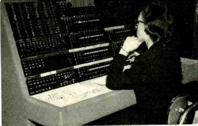
One operator at this switching center control console has American Airlines' complete Teletype services at her fingertips. Traffic may be diverted to intercept machines in the switching center when a station is out of order, and alarm bells and lights quickly pinpoint the malfunctioning station.
