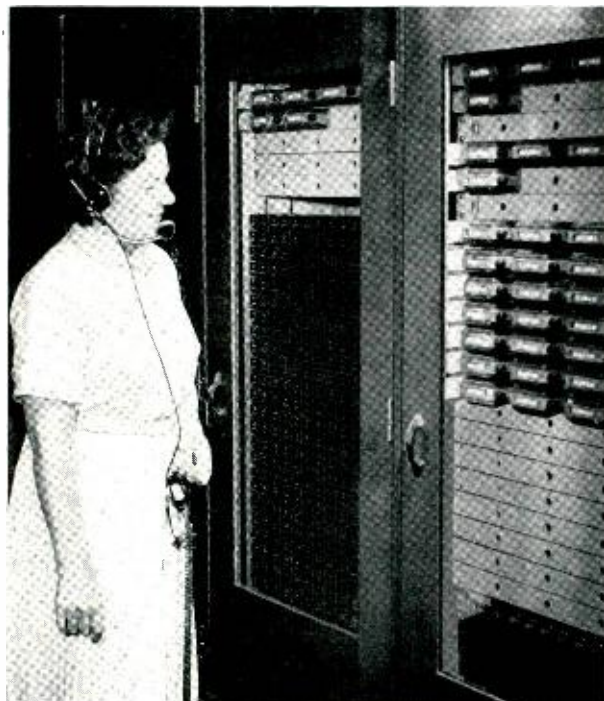
Fig. 2—The 14-type registers at the left and the electromagnetic counters on the right provide counts of equipment and trunk usage. A jack at the bottom of each bay permits the recording desk to be in a different room from the registers, the information being transferred by telephone.
