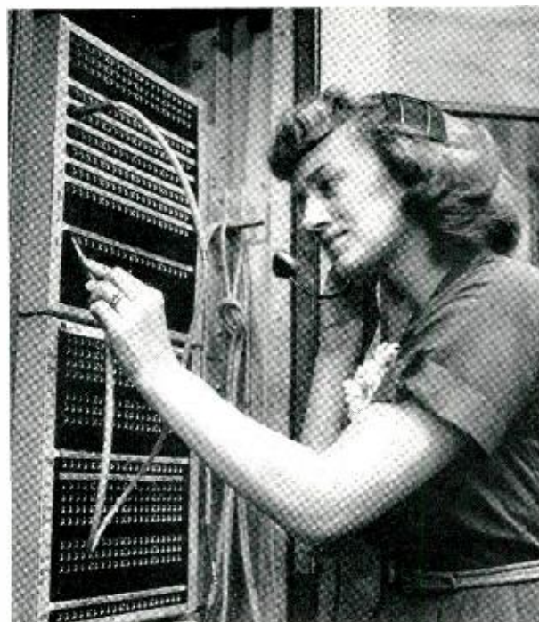
Fig. 1—The register patch bay provides interconnections between the registers and any desired circuit unit.
