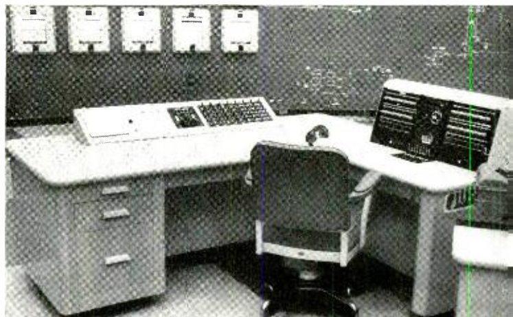
Fig. 1 — In the Bonneville installation, panels are “double decked” to provide a small working area.
