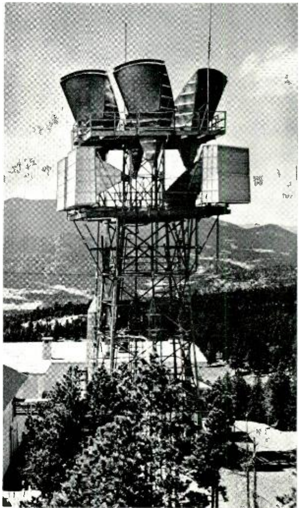
Antenna tower at Buckhorn Mountain, Colorado, microwave relay station. The 50-foot tower stands on a ground elevation of 8,306 feet. Mounted on it are both delay-lens and horn-reflector antennas.
