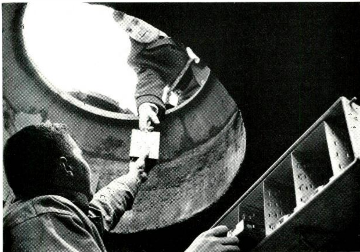
H. E. Brown, above, and M. S. Coldenhoff check out T1 System equipment in a Newark, N. J. manhole.
