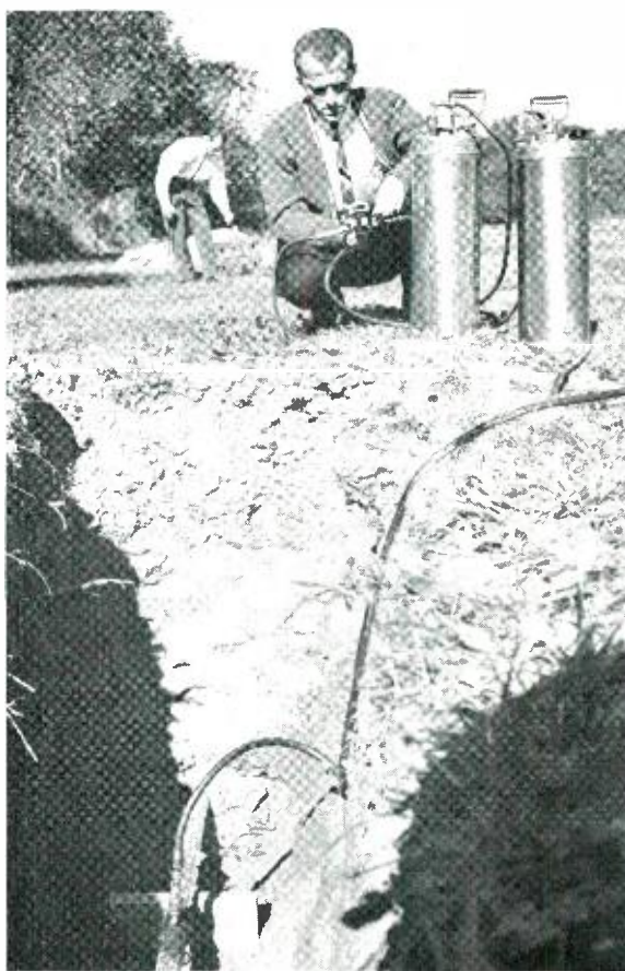
Author checks pressure gauge of acetone tanks while removing water from section of PIC cable.
