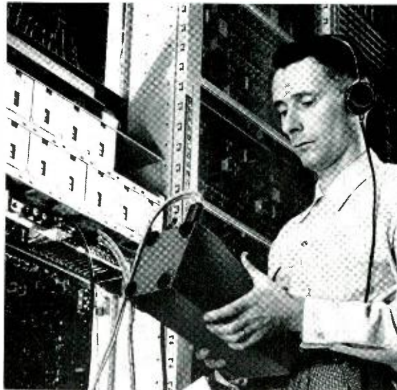
C. McGibbon of New Jersey Bell Telephone Co. checks E6 repeater at Westfield, N. J. office.
