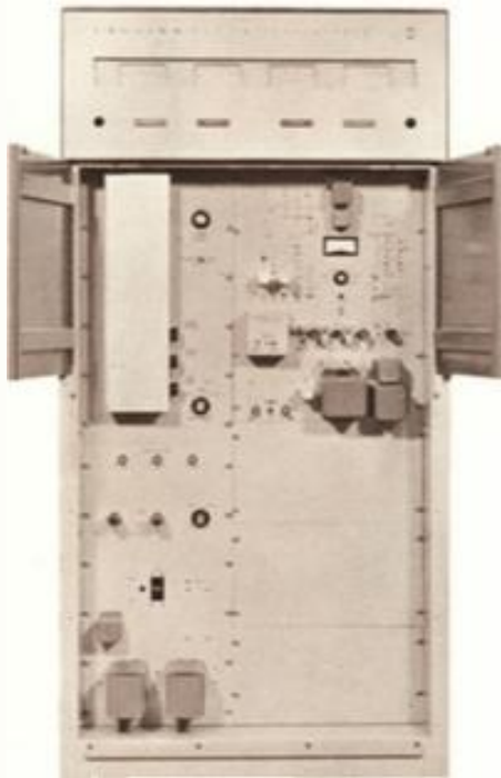
Driver front view, panel removed
