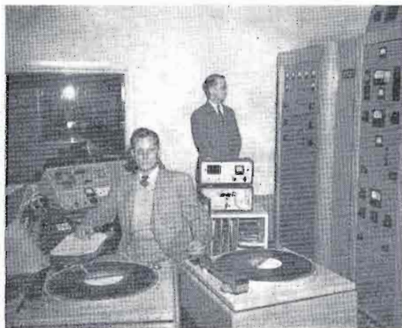
Complete businesslike installation of BC-250GY transmitter and associated equipment is well illustrated in this photograph from KPAT, Pampa, Texas.
