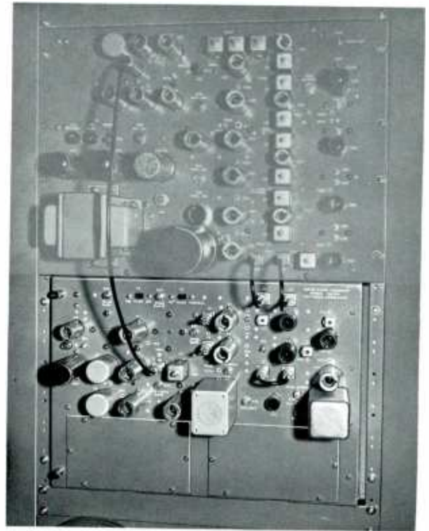
Top Unit — Gates "Cascade" FM Exciter. Lower Unit — M-6146 Stereo Generator.
