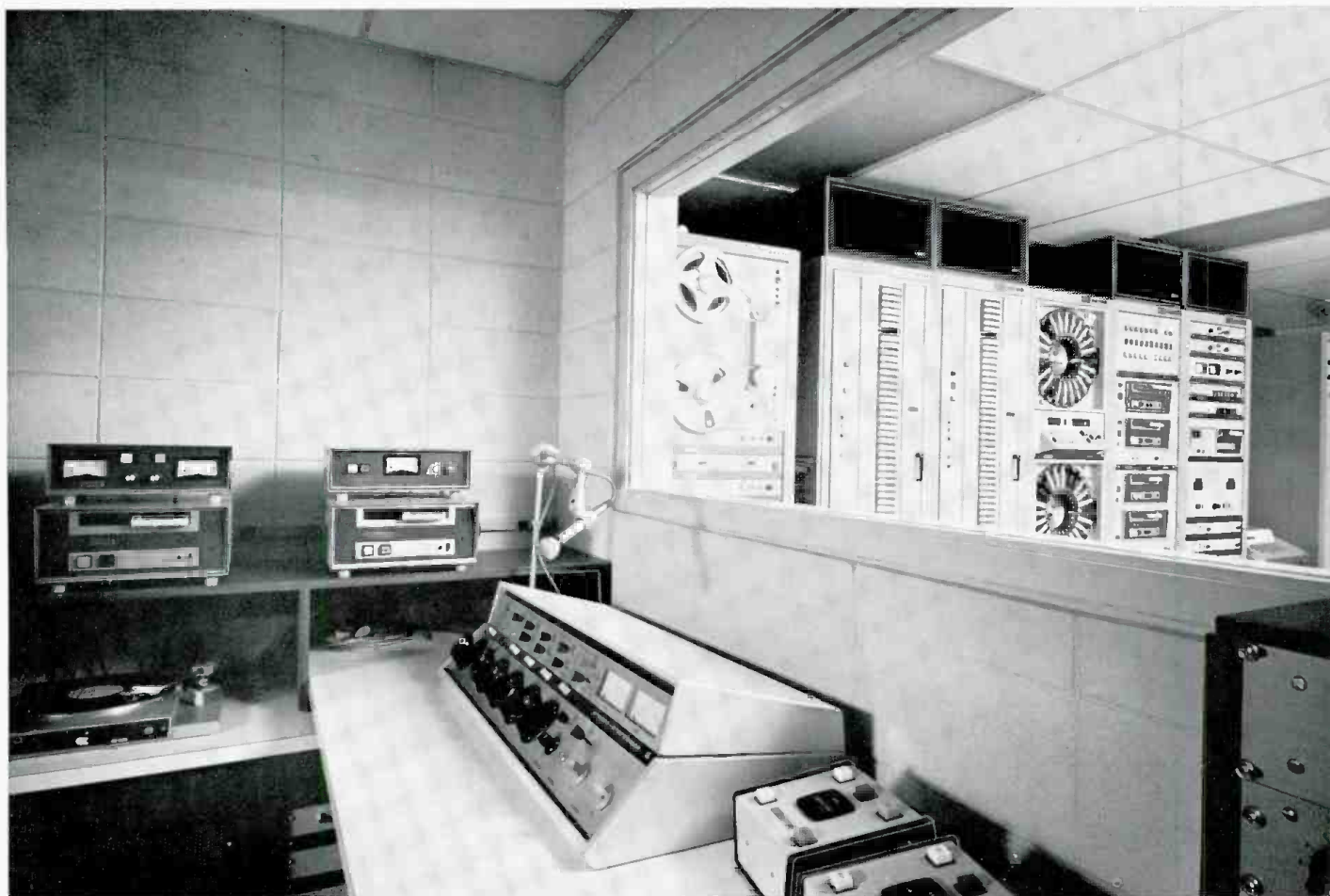
View of Gates' automation demonstration studio in Quincy, Illinois, showing a digital touch-control system. The studio is designed for station management and engineering evaluation of broadcast automation techniques.
