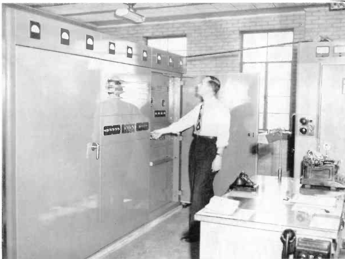
Above—BC-5B 5000 watt Gates broadcast transmitter installed at Radio Station WTAD, Quincy, Ill., CBS outlet and pioneer midwestern station.
