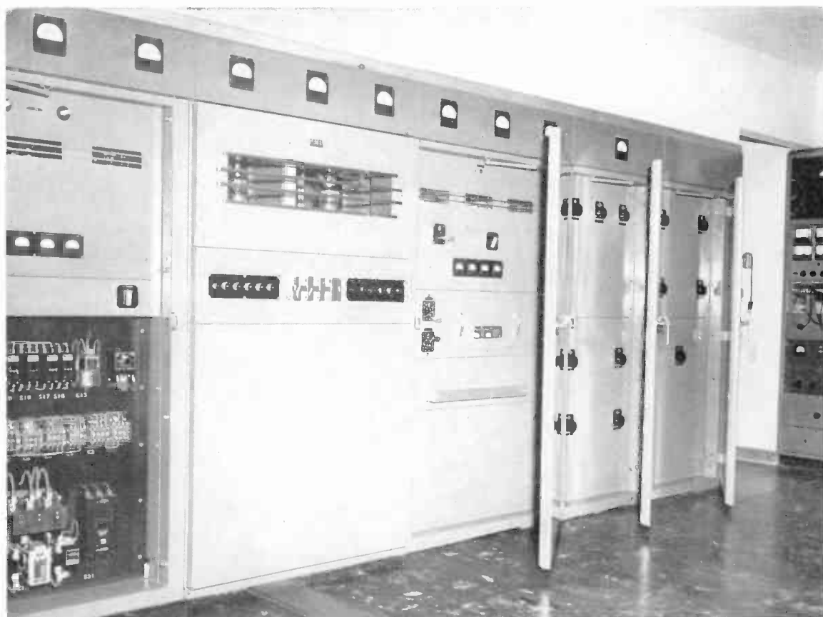
Below—Gates BC-5B 5000 watt equipment with five tower phasing equipment in matching cabinet at WENE, Endicott, N. Y.
