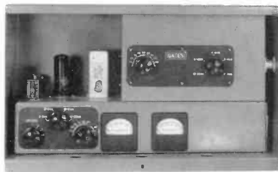
Front view of the oscillator-buffer section removed from transmitter. One of four crystals may be selected, and may be either temperature or non-temperature controlled.
