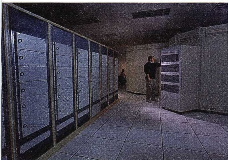
Advanced digital storage systems provide over 500 hours of on-line storage (left) and more than 50,000 hours of near-line storage.
